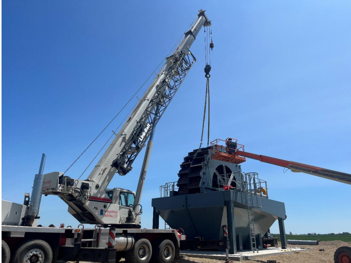
Jordan Eidsness is unhooking the top portion of the waterwheel from the crane hoist.
