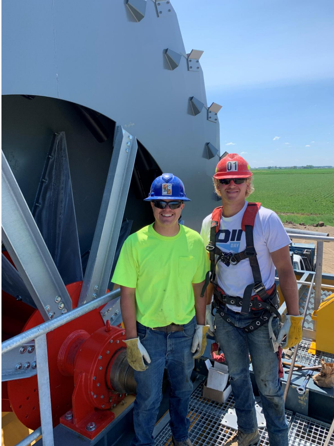
Ben Gadberry and Jaxton Schiller are busy working on the installation of the waterwheel.
