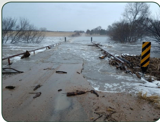
Nebraska road and bridge flood damage
