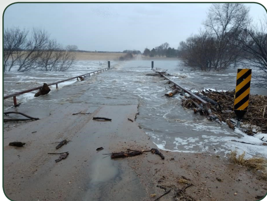
Nebraska road and bridge flood damage
